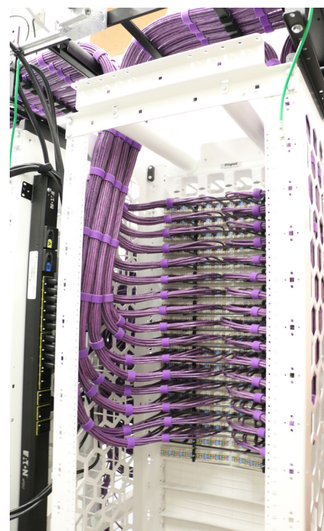
Angled Patch Panels
