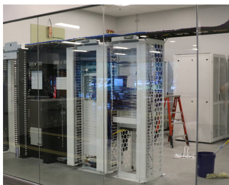
Glass-walled MTR Telecommunication rooms filled with seven 4-post Mighty Mo 20 racks and LX cabinets donated by Legrand
